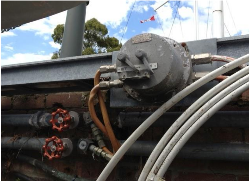
Remote Fuel Shut off Valve
